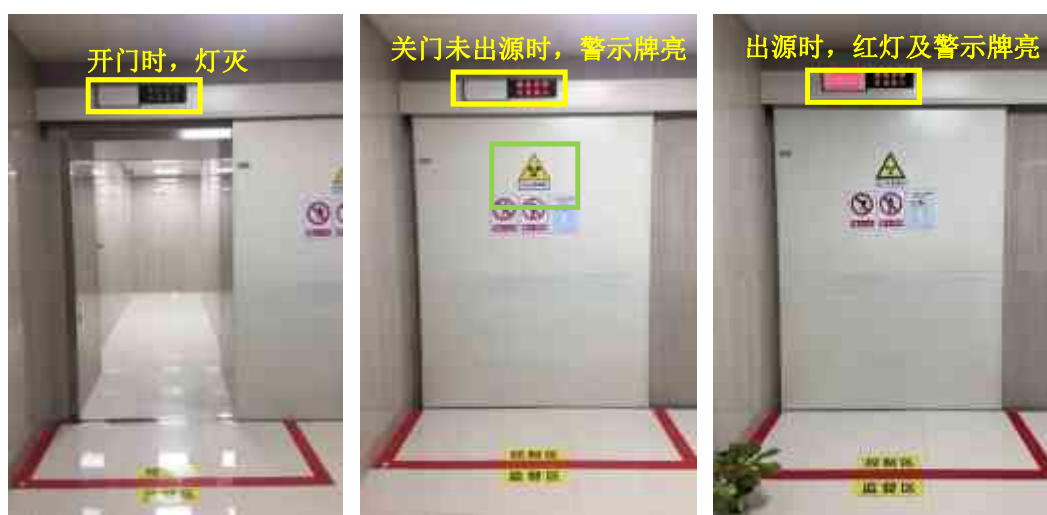
(c) 后装机房防护门
